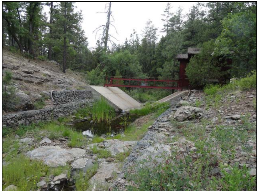
Figure 1. Stream-gauging weir, Beaver Creek Experimental Watershed. Photo courtesy Sharon Masek Lopez, Northern Arizona University
