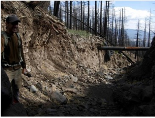
Figure 2. A municipal waterline is exposed from a 12-foot incision of a main drainage gully post-Schultz Fire.
